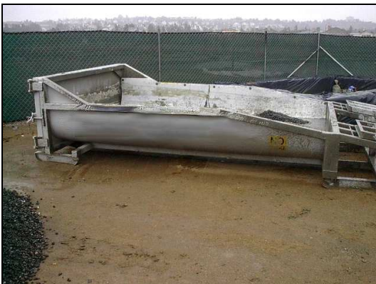
Prefabricated – reusable washout structure.
