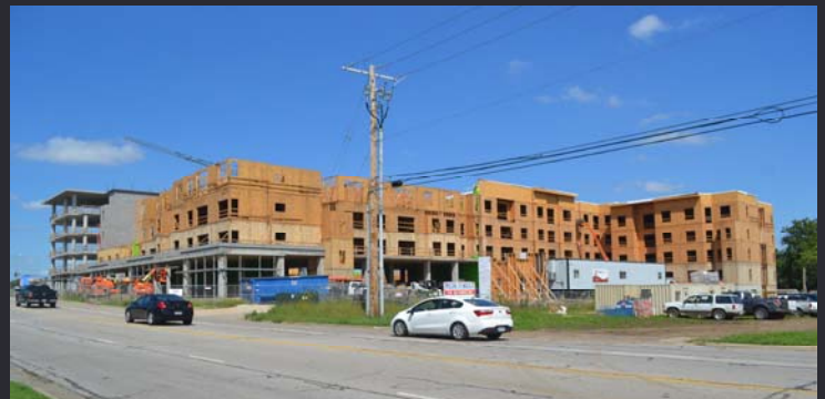
Avenue 80 is a $48 million redevelopment project at Metcalf Avenue and 80th Street. Adjacent to downtown Overland Park retail and restaurants, the mixed-use development is inline with the downtown form based code which focuses on the physical form of buildings and their relationship to the city street in order to create a mix of uses in a walkable environment. This project is one of four large mixed-use projects being constructed in downtown Overland Park beginning in 2015.
